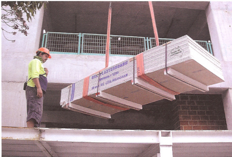
A photo supplied by the CFMEU showing a worker operating at height on a surface without edge protection.
